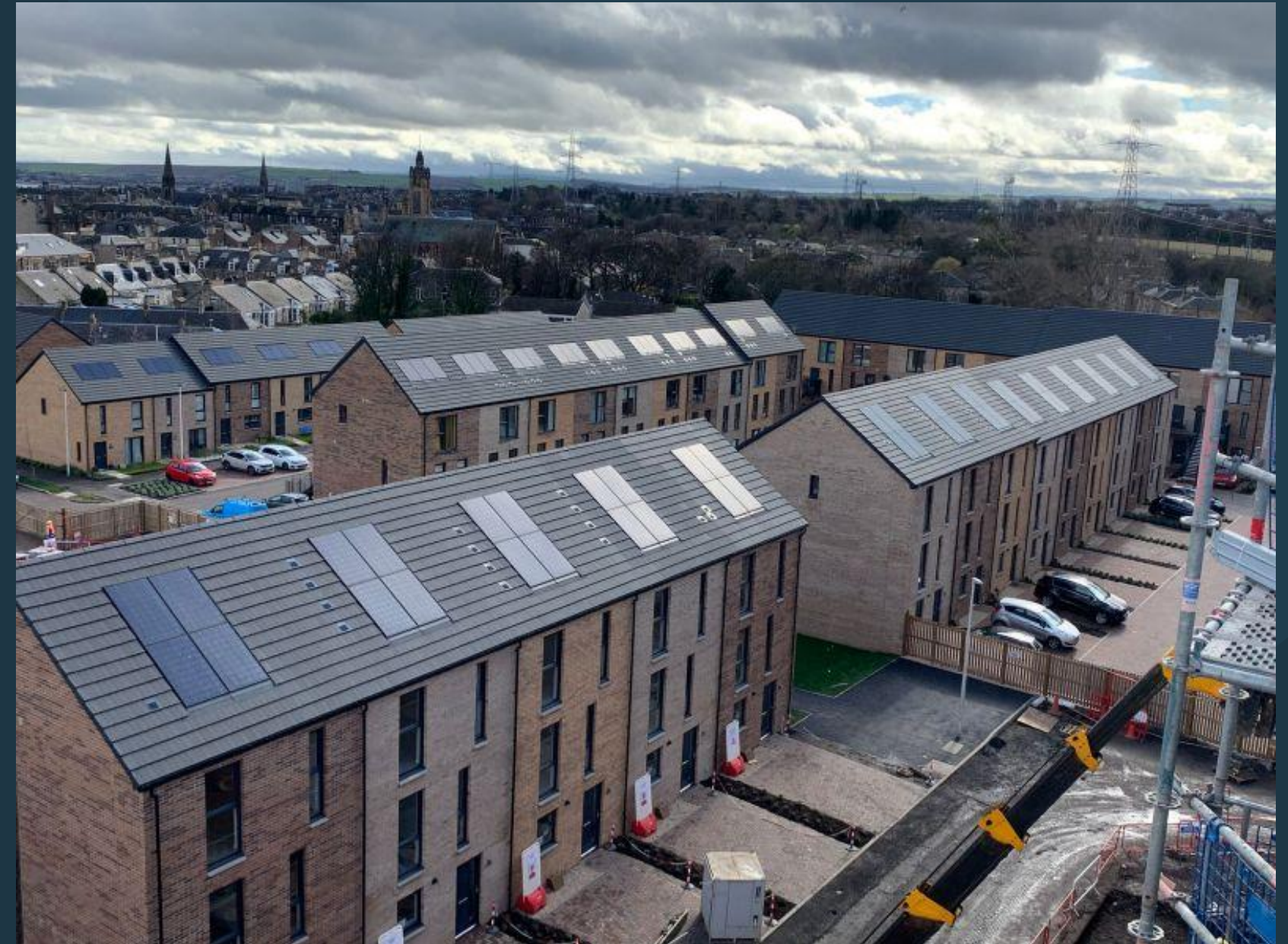
In-Roof Solar PV
